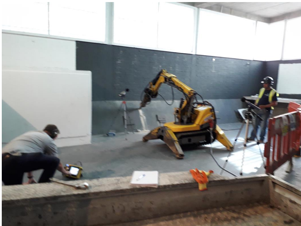
A3.15: Test No. 15 – Brock Chipping on Slab, Lobby, Ground Floor.
