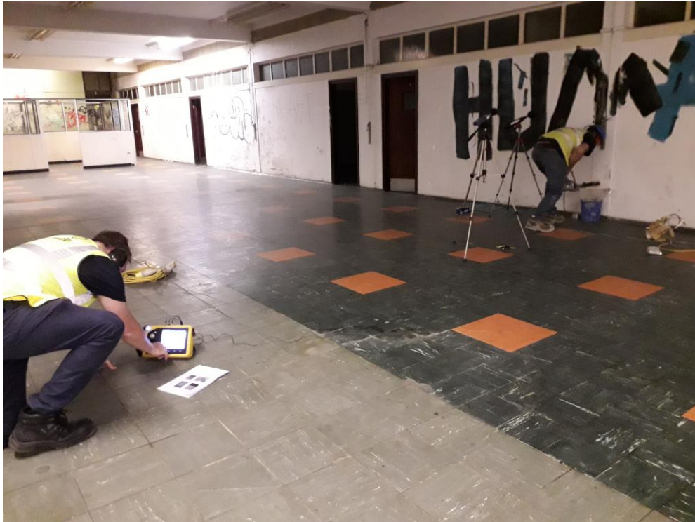
A3.3: Test No. 3 – Boring Holes to Coring Column, Main Room, Ground Floor.
