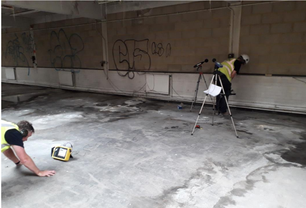
A3.9: Test No. 9 – Boring Holes to Coring Column, Main Room, First Floor.
